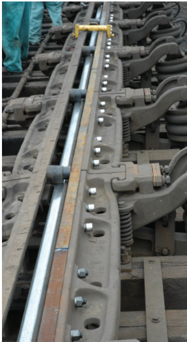
Left: CSX has used Tracksure to secure retarder brake pads in one of its hump yards.
